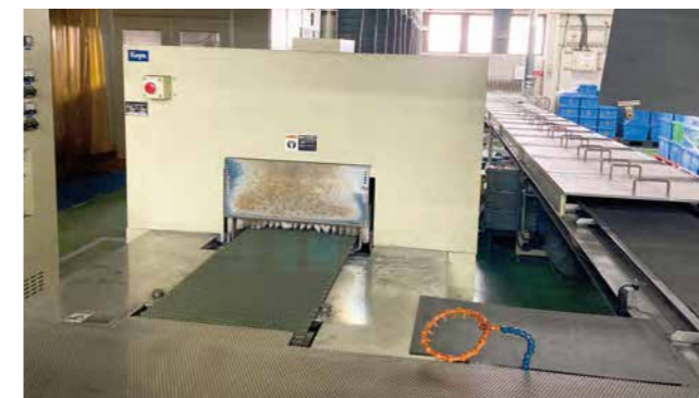
3D thermoforming facility / serial heating machine
